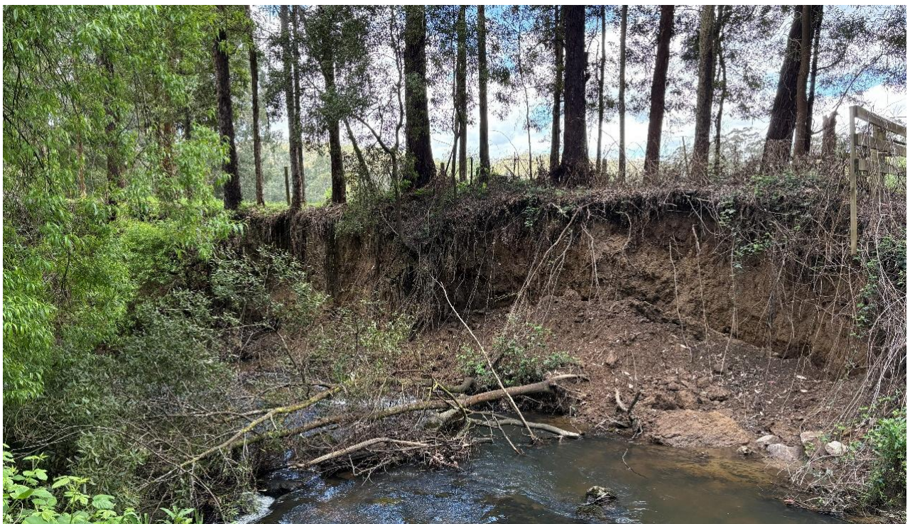
Figure 10. Bank erosion at Lardner Creek stream depth gauge
