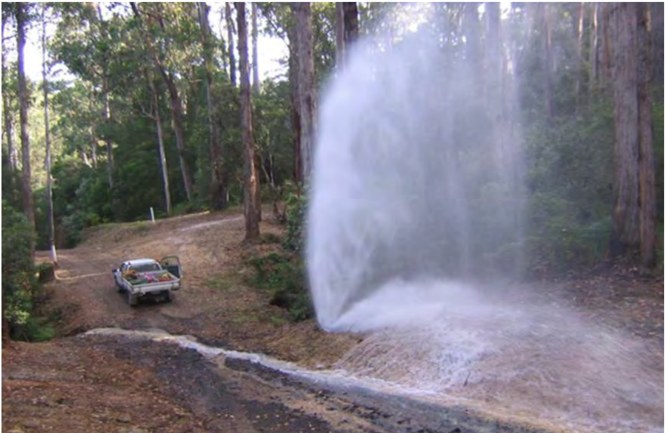
Plate 1 Example of a pipeline burst incident on the existing Colac Pipeline
